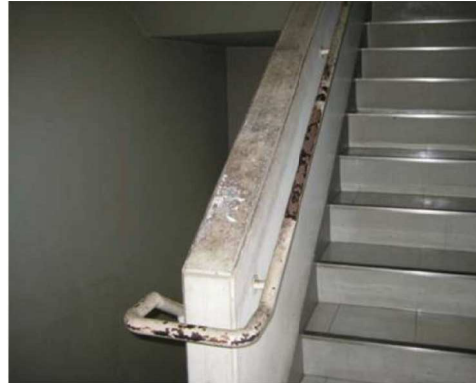
階段手摺の腐食
